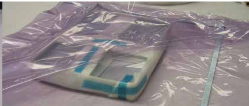
Figure 2. Breather fabric is attached to the glass and across the flat surfaces using Solvay blue FLASHTAPE 1, 25mm (1in) wide. Note that the material must extend to the underside of the vacuum port.
