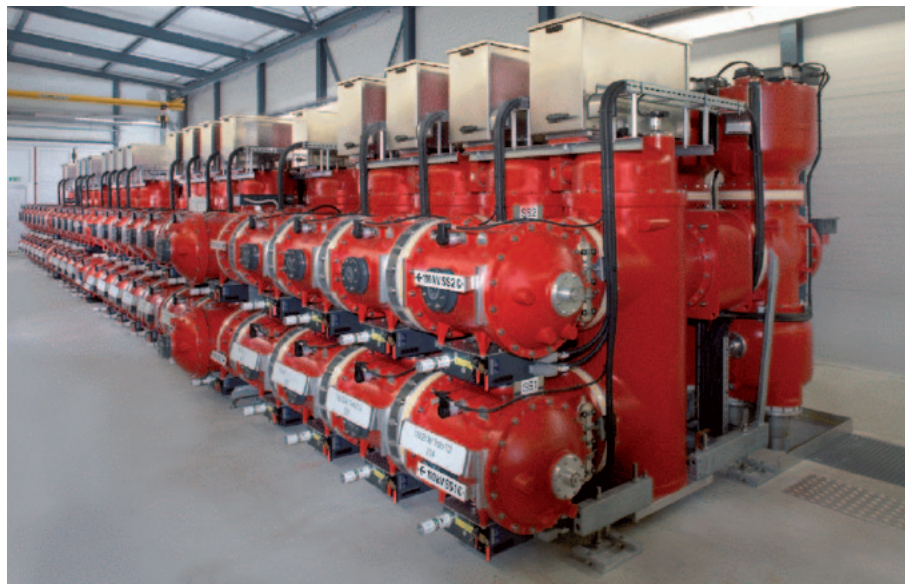
Fig. 7 GIS substation, 145 kV (Alstom Grid, Switzerland)
