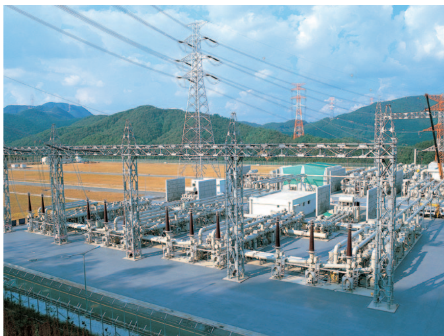
Fig. 3 Gas insulated, high-voltage switching station, 800 kV (Hyosung, South Korea)
