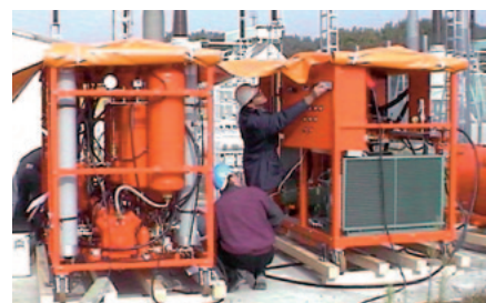
Fig. 9 \text{SF}_6/\text{N}_2 -membrane-separation plant with condenser unit
