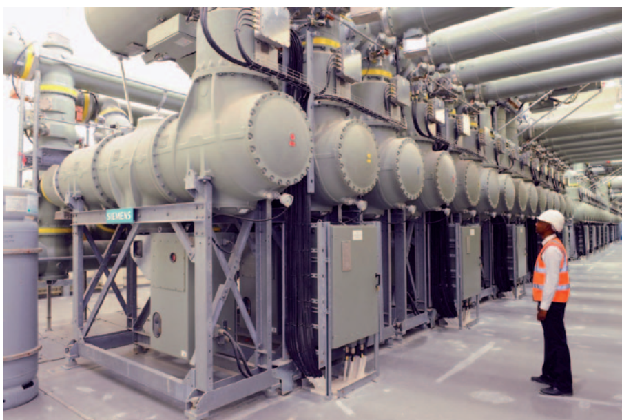
Fig. 1 SF 6 -insulated, high-voltage switching station, 500 kV (Siemens, Germany)
