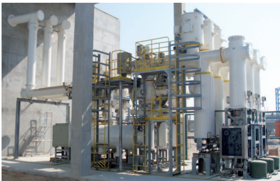
Fig. 5 Gas insulated, high-voltage switching station, 420 kV (Hyundai, South Korea)
