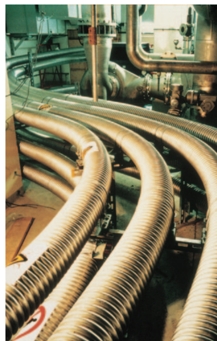
Fig. 16 \text{SF}_6 -insulated high-voltage cable in the JET nuclear-fusion plant (kabelmetal electro, Germany)
