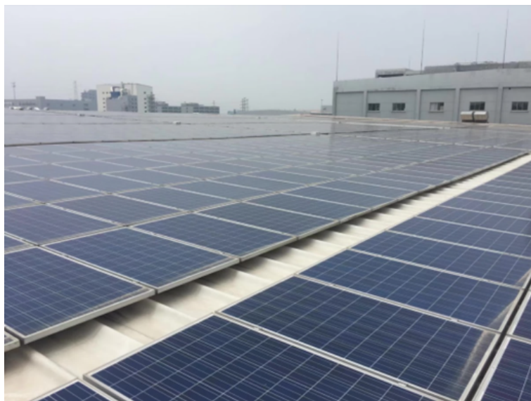
3TREES' BIPV solution incorporating Solvay's UV/thermal stabilizers. (Photo: Solvay, PR044)
